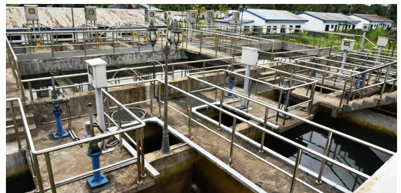
Lobe drinking water treatment plant, South region
